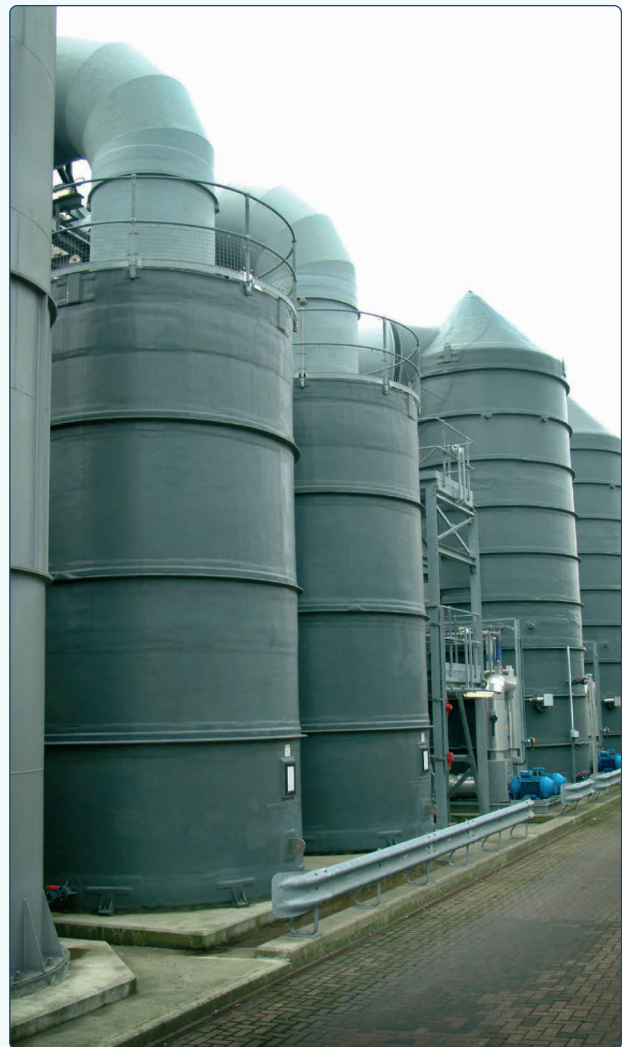
Combined Technology Odour Control - Carbon and Scrubbing
