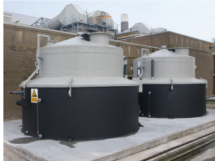
15,000 Litre Dual Minitank, uPVC/GRP tank and pp bund - Kilroot Power Station, Northern Ireland. Tanks are storing 12-15% Sodium Hypochlorite.
