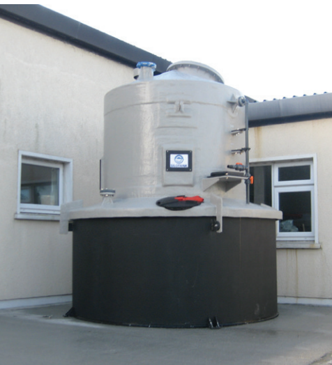
20,000 Litre Dual Laminate Minitank, cPVC/GRP tank c/w PP bund - Ballinasloe WTW, Ireland. Tank is storing 98% Sulphuric acid.
