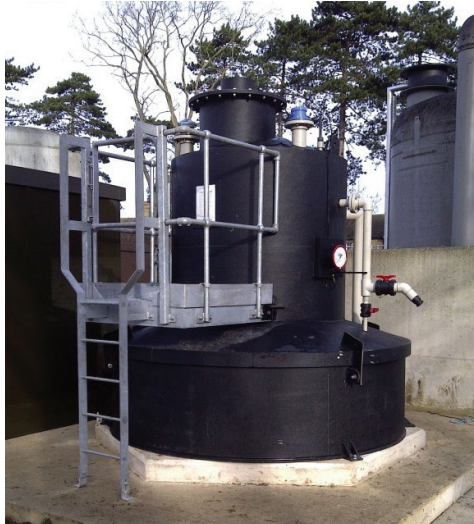
2,500 Litre Polypropylene Minitank, PP tank c/w pp bund including access platform - Forstall WTW, South East Water, England. Tank is storing 23% Sodium Bisulphite.
